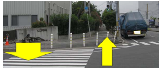
Fig. 2 Subsidence in liquefied private land that induced uplift deformation in public road
