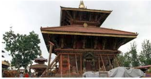
Figure 22. Two-tiered pagoda after the earthquake protected by scaffolding.
