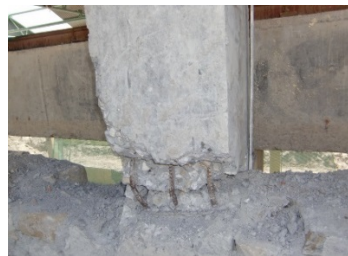
(b) Rupture of reinforcement bar
