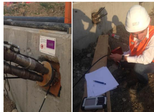
Figure 9. Images from work site measuring force in ground anchors during tensioning and lock-off
