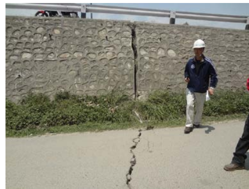
(b) Ground cracks
