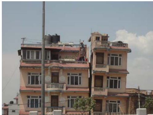
(b) Tilted apartment building
