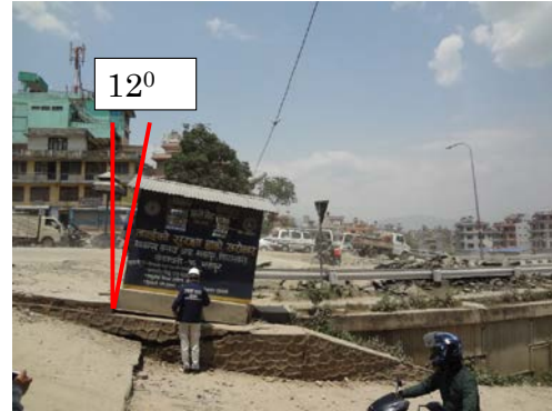
Figure 6. Slope failure in the Kathmandu side
