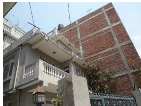
Figure 10. Settlement and tilting of buildings resulting from ground fissuring.
