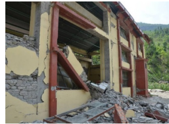
(a) Wall collapse on riverside
