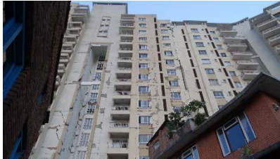
Figure 30. A typical case of damage to tall buildings.
