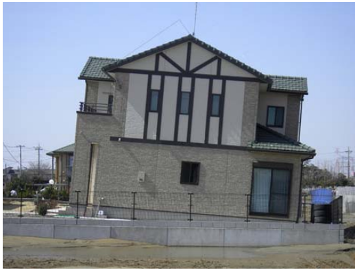
Fig.1 Liquefaction-induced tilting of house
