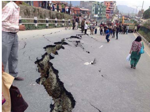
(a) Subsidence of the access road
