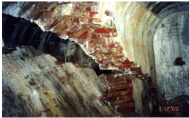
Figure 7. Collapsing cellar wall behind east loggias.
