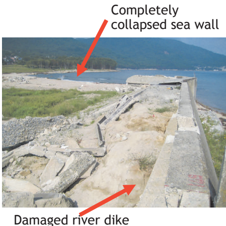
Figure 6. Damaged river dike in Yoshihama area
