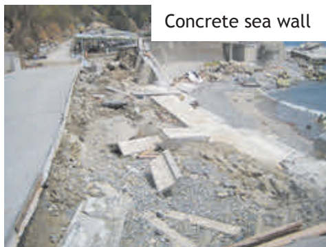
Figure 2. Collapsed sea wall in Okirai
