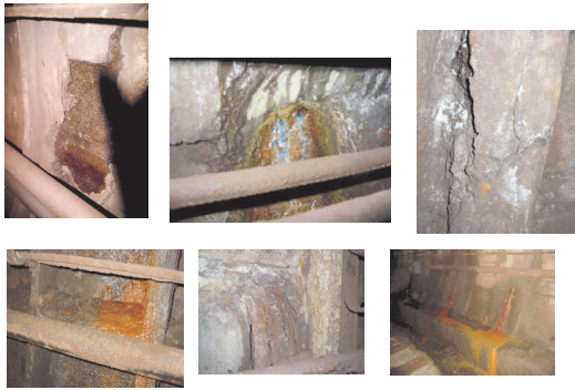
Figure 8. Active biocorrosion of reinforced-concrete tubing of Saint-Petersburg Metro systems
