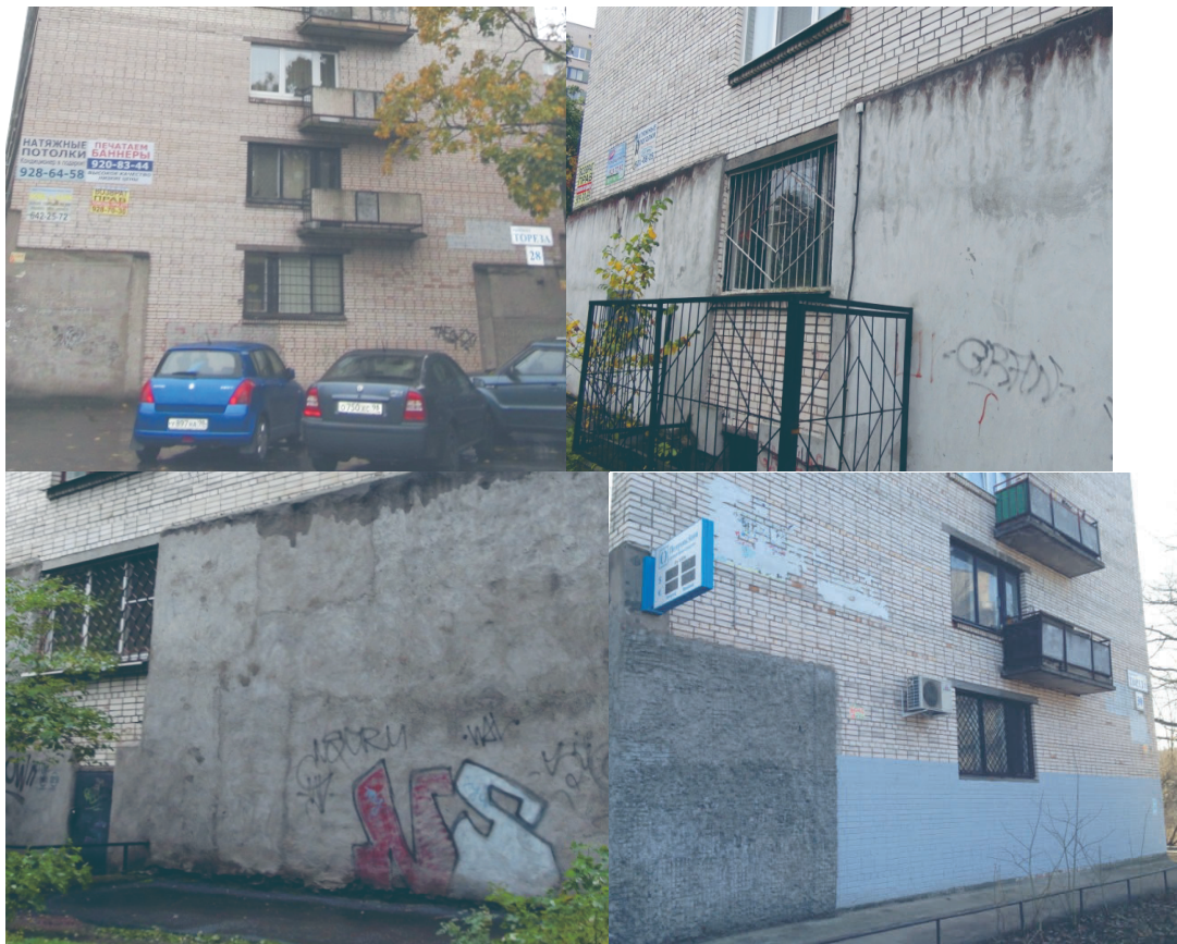
Fig. 30. Reinforced concrete strengthening patches in edge zones of gable walls on the building of the standard series u -5733.
